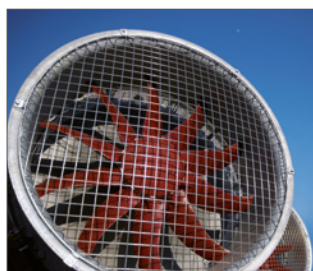
HVAC AND PUMP SYSTEMS
